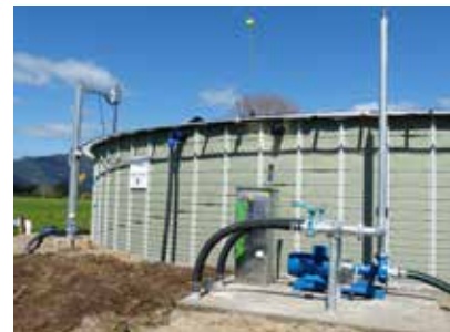
Submersible Stirrer and Above Ground Lifting Frame on KlipTank.
