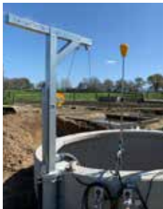
Submersible Pump and Lifting frame on Sump application.
