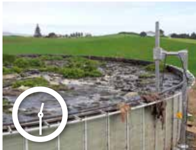
Submersible Stirrer and Over the Wall Lifting frame on Tank application. Time Lapse: 0.5hr and 3.5hr.
