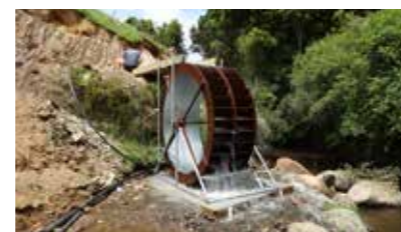
CS_PUM01 8' x 3' Yardmaster Water Wheel. Water accessed via farm creek dam and delivered via PVC to wooden flume
